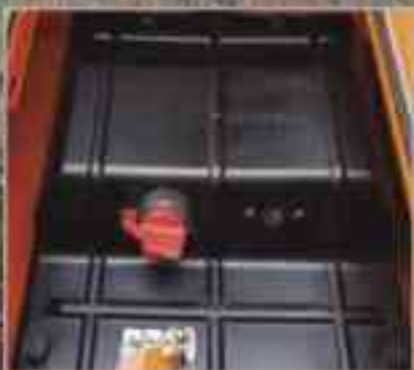
Battery cut-off switch
