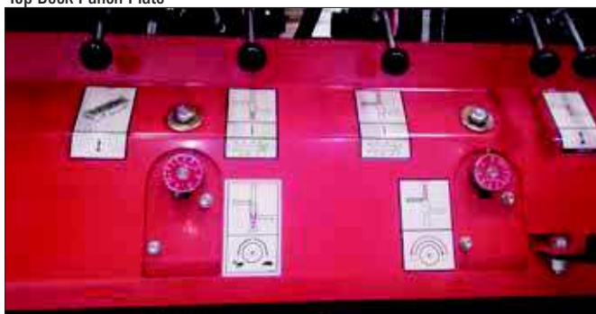
Powerunit - valve bank
